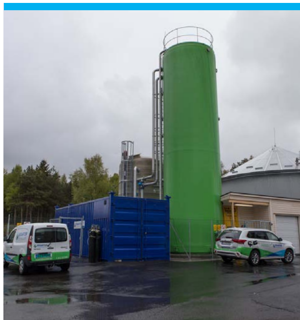
Turnkey HyVAB project delivery by Biowater
